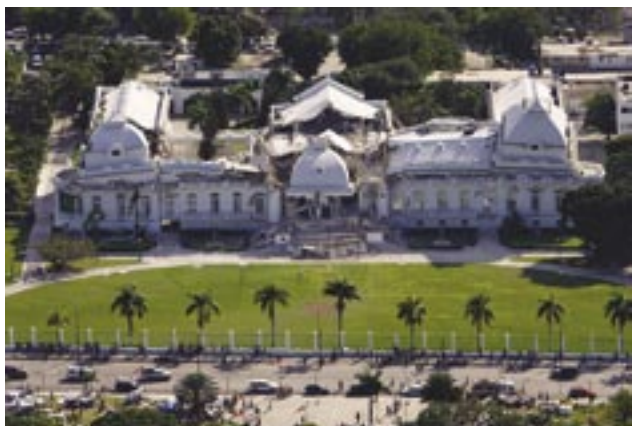
The Haitian national palace shows heavy damage after the earthquake. Getty Images/United Nations/Logan Abassi
